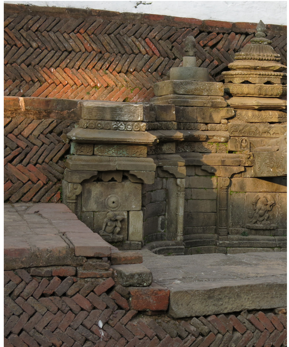
North Hiti. Few bricks in fish tail pattern were missing behind the centre of the hiti on 4th level, on the left side of the hiti on the 3rd level and just below the steps on 2nd level plinth. Photo: Jan., 2013.
