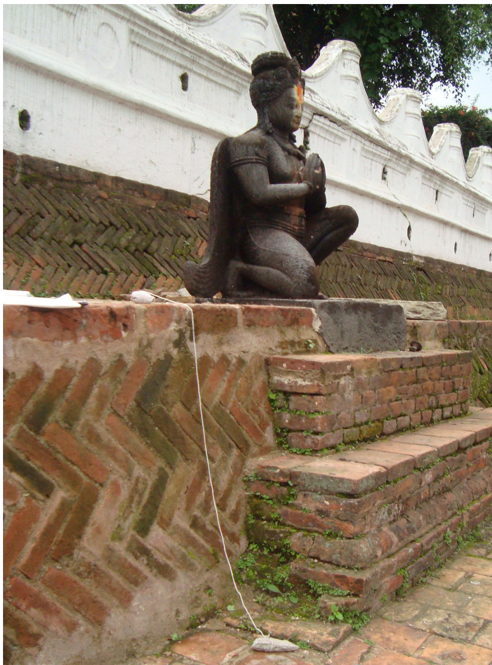
A small section of 3rd level plinth was repaired recently in lime surkhi mortar on the right side of the Garuda. Lime surkhi mortar was rendered heavily on the joints and does not match the older sections, built in mud mortar. Three sides of the base is sunken on the 3rd plinth, which is logical to lift to make the stone base visible from all four sides. Photo: Jun., 2013.
