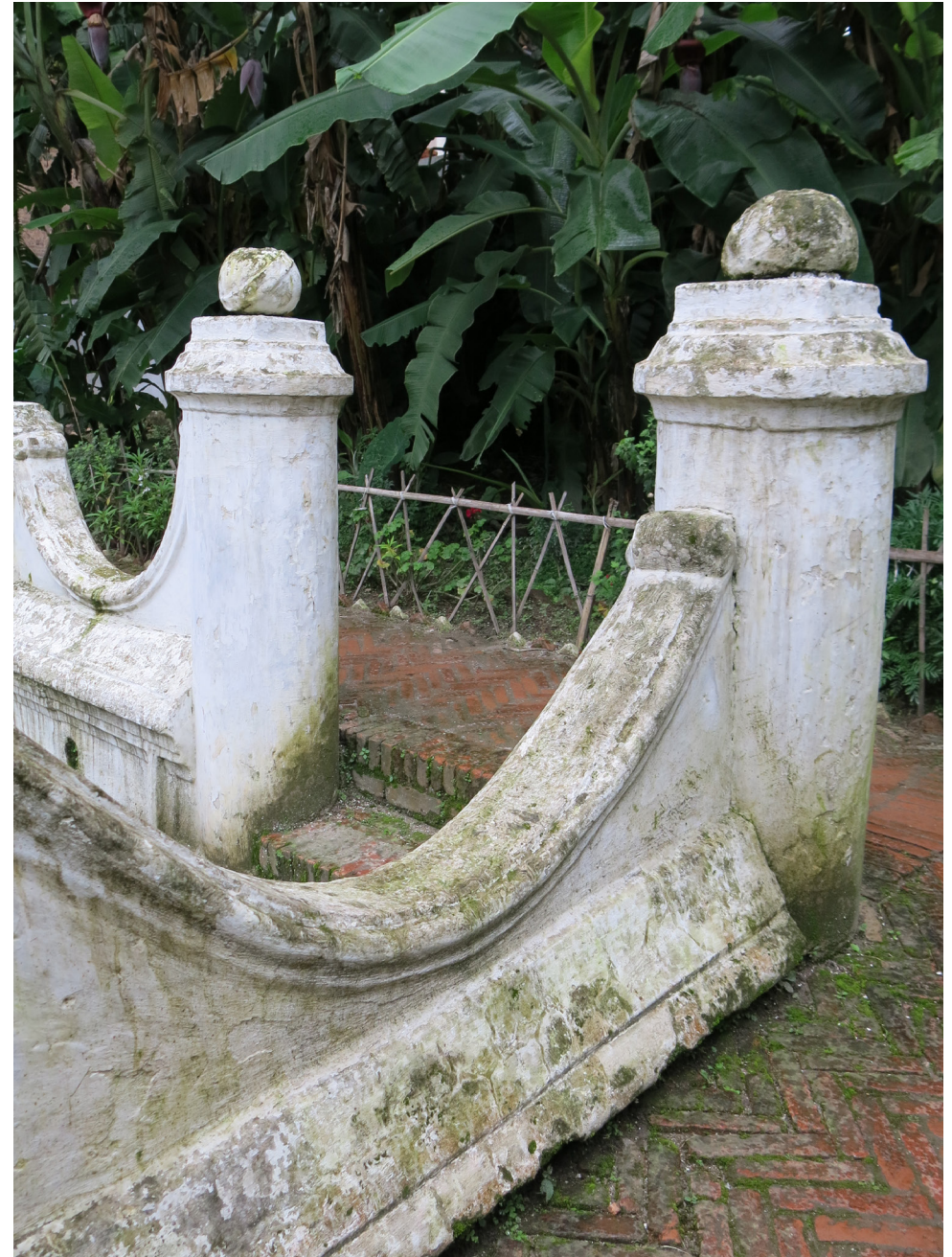
One of the top of the pillar ornament on the south stair should be reproduced to match the existing pillar on the other side. Photo: Jul., 2013
