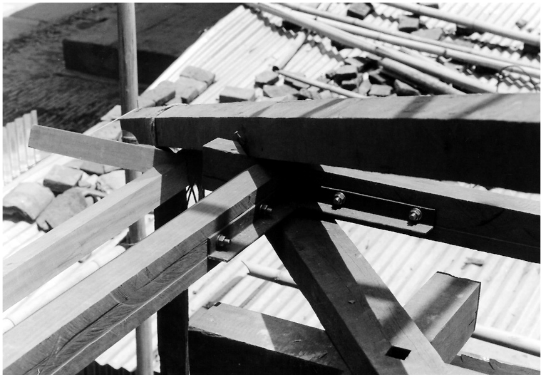
On the steel angle, nuts and bolts are used at the joint of the purlin, tying them together acting as one unit in the event of a seismic movement.
