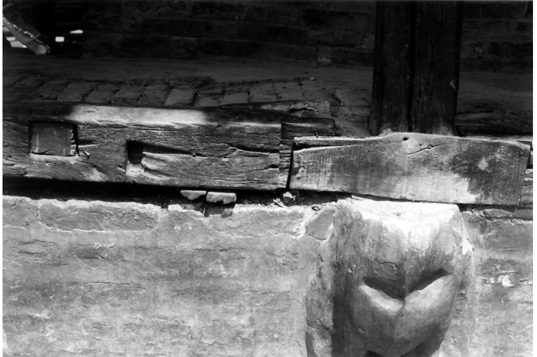
Damaged condition of lakasi (base of arcade pillar).
