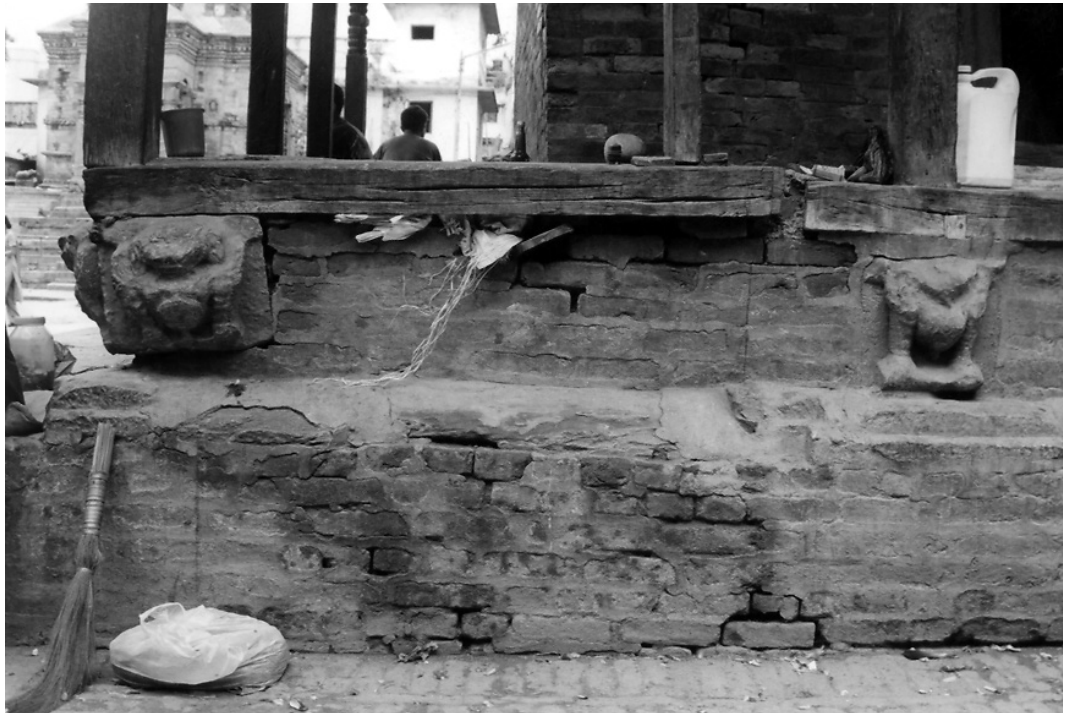
Damaged condition of the plinth level wall where the outer plinth does not exist.
