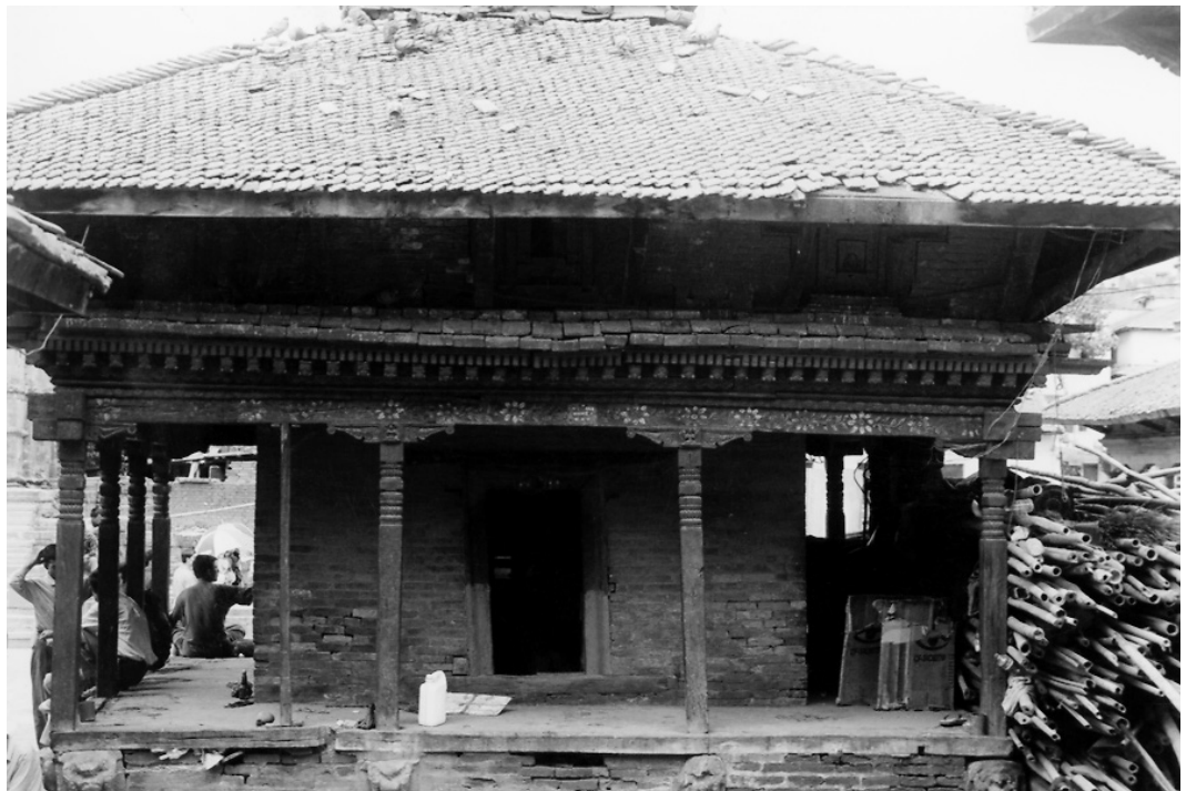
A southern view of the Temple showing the poor condition of the arcade and lower roof.
