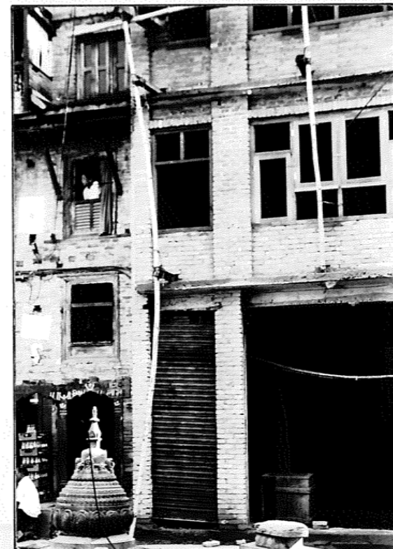
Tamrakar house, Haugah: the 12 ft. ground floor ceiling height is illegal. Notice how the new ground floor steel rolling shutter (also illegal) reaches the same height as the first floor window of the traditional house to the left.
