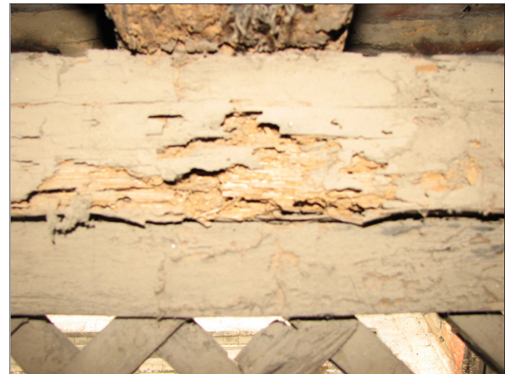
rotten decay at 2.5.
