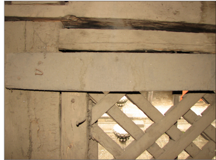
low grade repair at the frame work 2.5.
