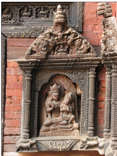
2.7.N.06 Frame -after the earthquake, Statue and tympanum-original.
