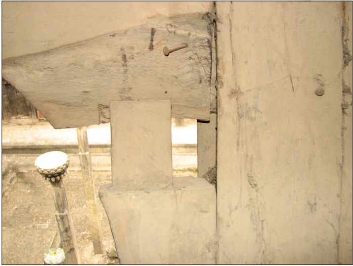
damaged frame joint at 2.5.W.06
