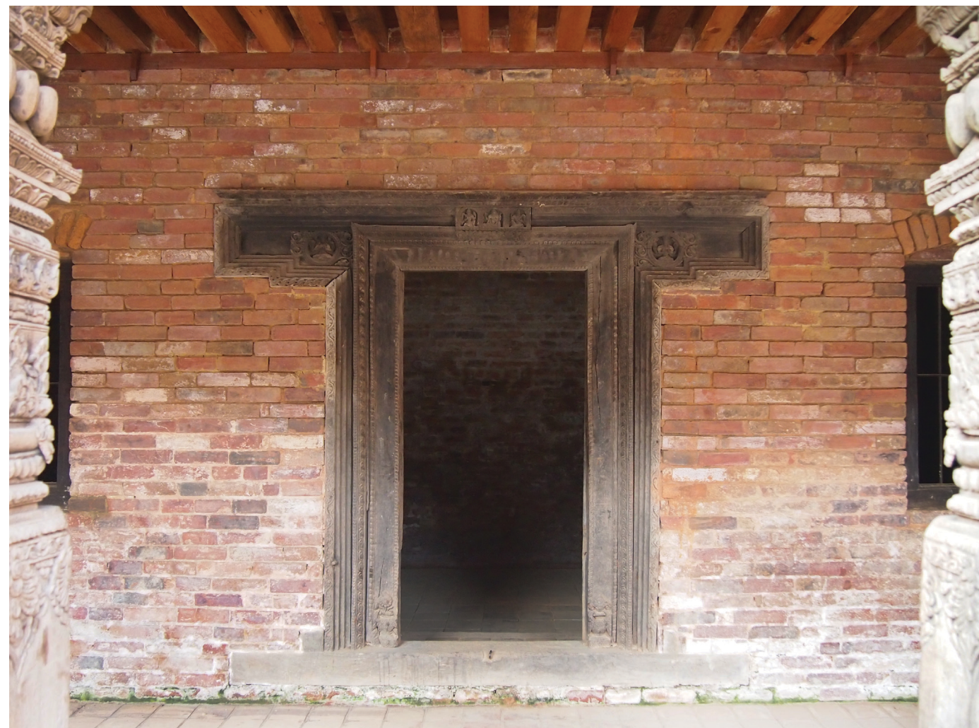
Entry to Gallery 00 Efflorescence indicates rising damp and transport of salts to the brick surface. The wall will require continued cleaning. Signboards for the documentation gallery will be mounted on either side of the door. April, 2012
