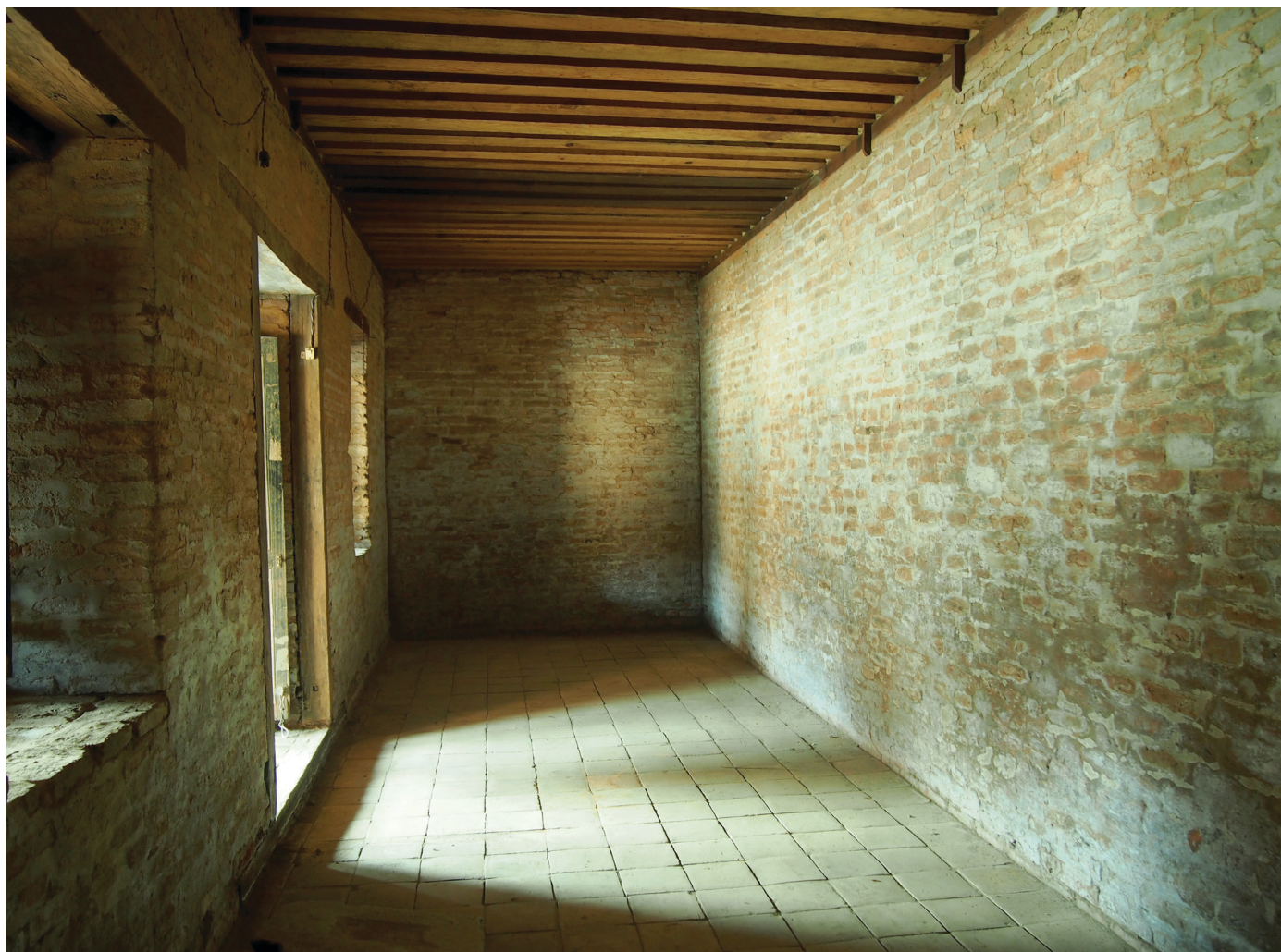
Gallery 00 after restoration Rising damp affects most ground floor walls. It is not recommended to plaster the walls but rather to treat the surface with a brick color tinted lime wash. The documentation panels will be mounted on water-proof plywood installed at a distance of 4 inches to the walls. Photograph April, 2012
