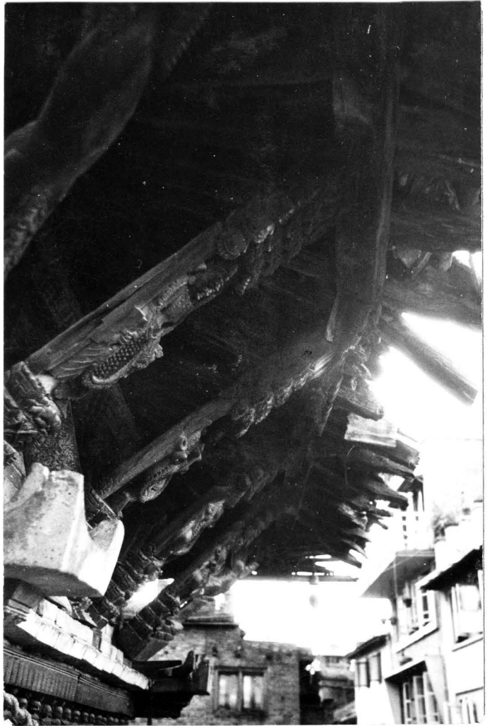
Right: Eavesboard already lost and rafter ends rotted off, Upper pagoda(lower of two roofs) , south elevation. August 1993. Below: Only a few metal strips hold a damaged eavesboard on west facade, upper pagoda (lower of two roofs).August 1993.
