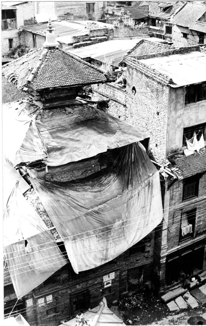
Left : Gap between bottom of pinnacle and roof tiles. August 1993.
