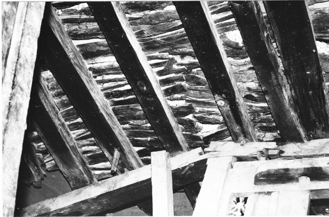
Timber lath above pine rafters has transmitted dampness from mud to rafter. Principal facade, August 1993.
