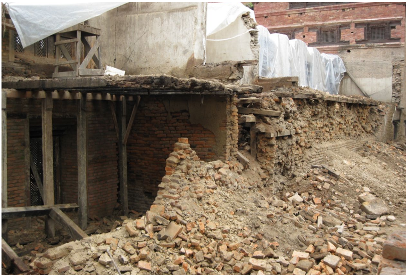
October 2010: The completely dismantled east wing, showing the severely damaged timber joists. None of the structural timber components could be reused for the restoration.
